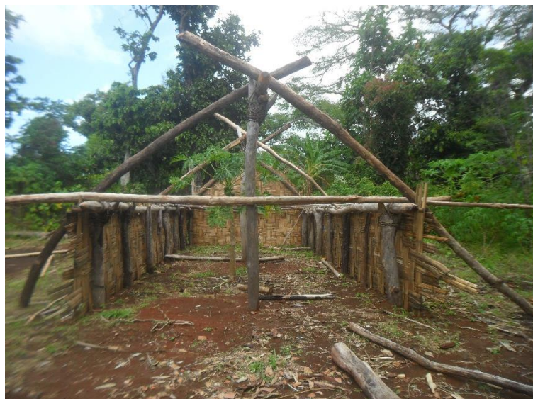
Construction of South River's evacuation centre has begun – and the whole community is getting involved to make it happen. © Marie Toto/CARE
