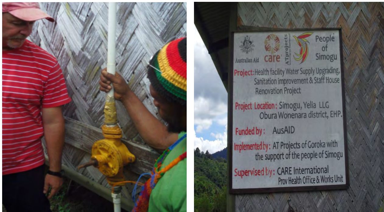
Figure 11 – Broken water pump at Simogu and CARE / AusAID signage
