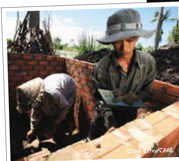
Vaan Van Tsang builds a latrine for his family in Vietnam with materials provided by CARE.
